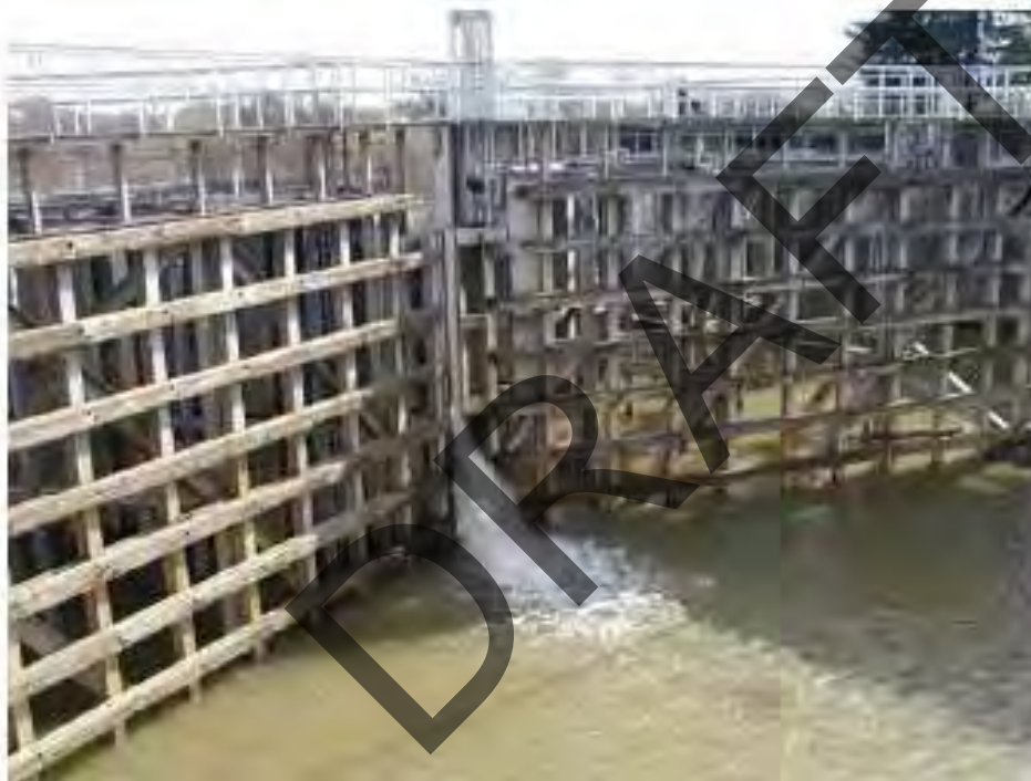
Exhibit 37: Sacramento River Water Leaking through Western Sector Gate
